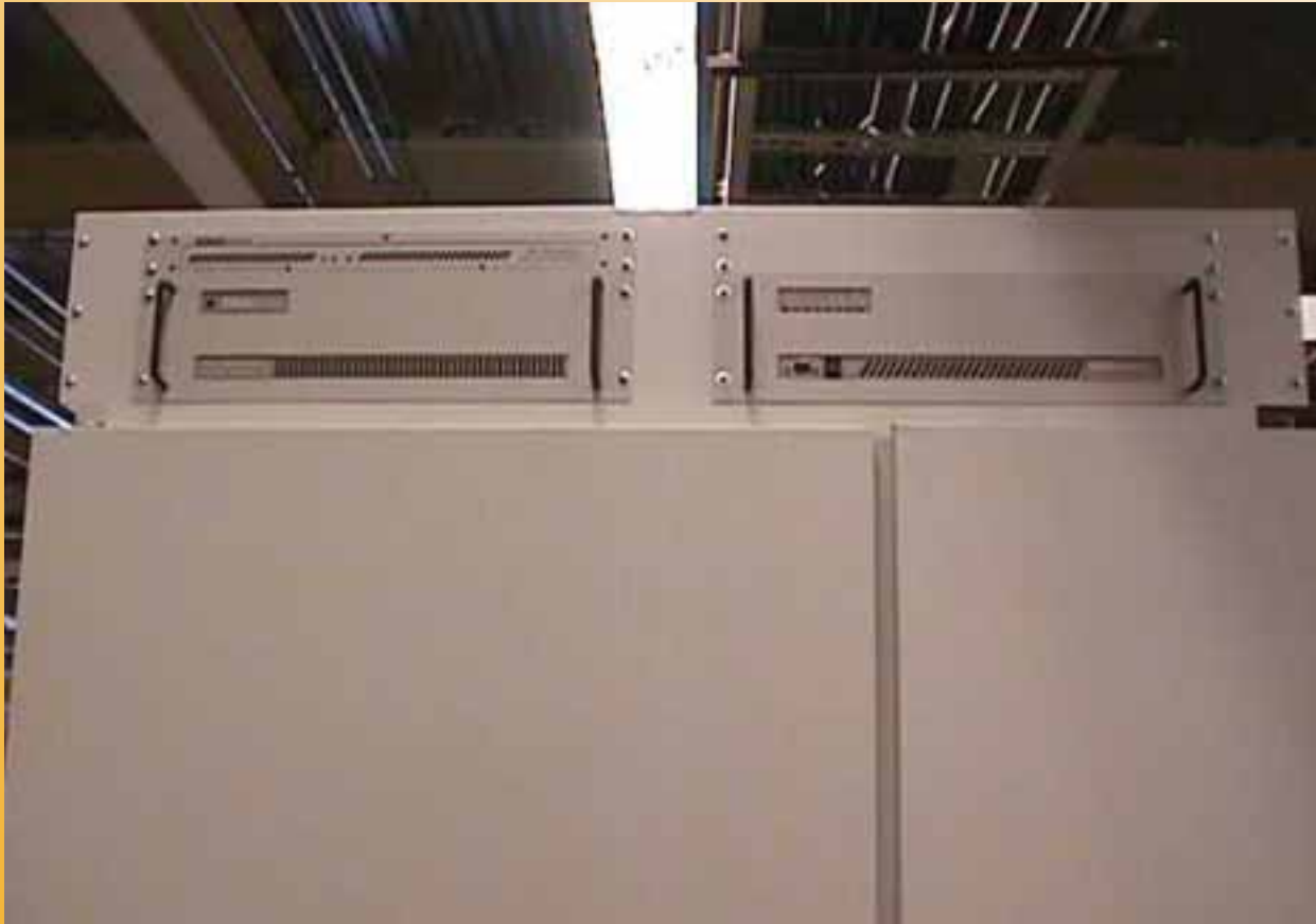
Mounted on top of MGE 6000 Cabinet
